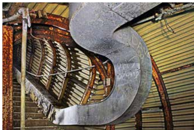
Original ventilation trunking still in place at the bottom of the entrance stairs. Photo Richard Crowhurst / Corvidae Ltd First World War success
